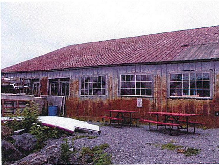
Contemporary photo showing present window configurations. Note the shifting of the window frames because of the settling structure.
