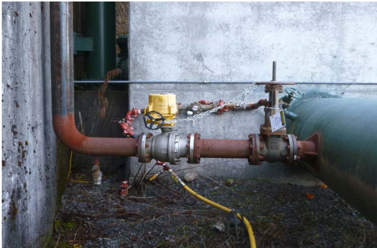
Figure 1 – Existing 6” Supply Line to Filter Forebay tapped off 36” PMFU Penstock Pipe. (Manual isolation gate valve followed by AWWA C507 Class 150 (to be verified by CBS?) stainless steel, full-port ball valve.)
