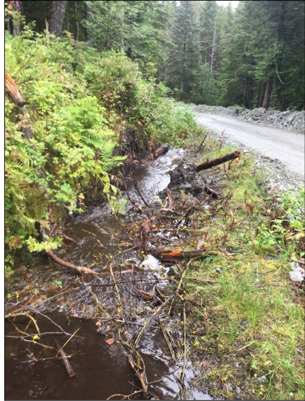
Figure 2.–Drainage downstream and adjacent to Comet Beach Road.
