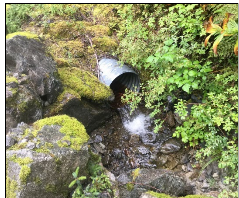
Figure 4.–Perched culvert downstream of fish capture locations.
