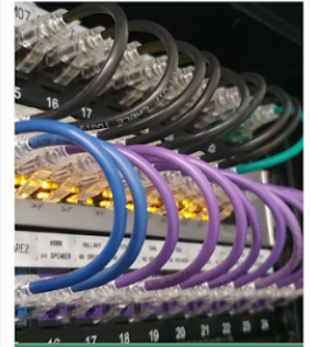
PATCH CABLES COLOR CODED & LABELLED
