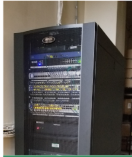
ENTERPRISE RACKS SECURED & ACCESSIBLE
