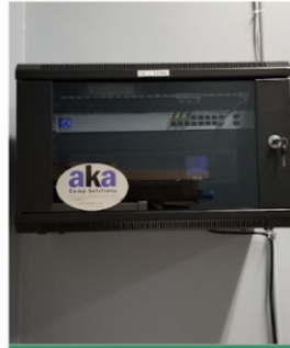
IDF RACK MOUNTS SECURED INSTALLS
